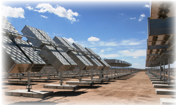
The 2-megawatt Solar Array Farm at the Eubank Landfill.
